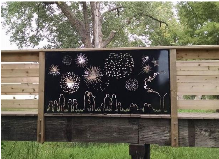
Finished bridge with first panel installed. First panel represents the impact Randolph Independence Day Celebration has on the community.
